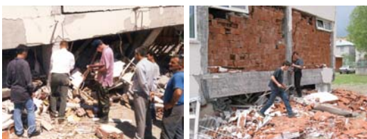
Figure 2. Documentation of structural damage by the engineering group of German TaskForce (EDAC staff) after the (left) 1999 Kocaeli and (right) 2003 Bingöl earthquake.
